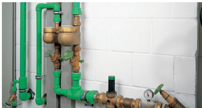
From the house connection station, cold water distribution, boiler connection and hot water distributor...
