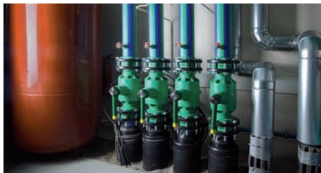
Flange connections and transition joints enable the connection of all components to the central heating system and on the floor.
