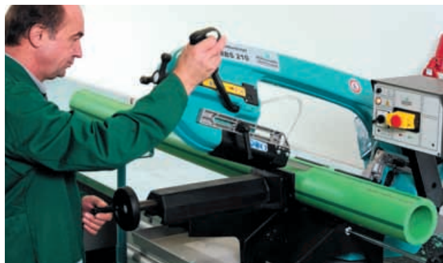
Before welding, the 160, 200 or 250 mm pipes are cut into the required lengths
